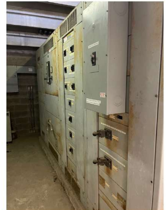
East Electrical Room
