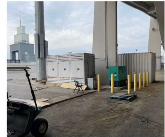
East Tower Generator
