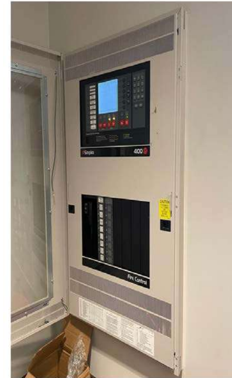
East Lobby FA Control Panel
