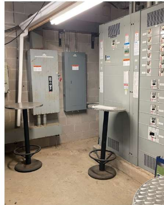
West Electrical Room
