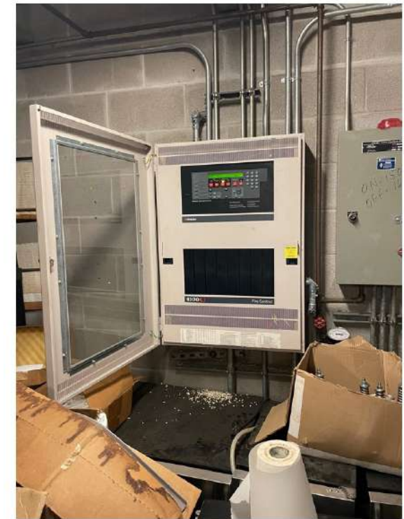
Electrical Room FA Control Panel
