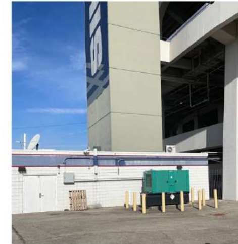
West Tower Generator
