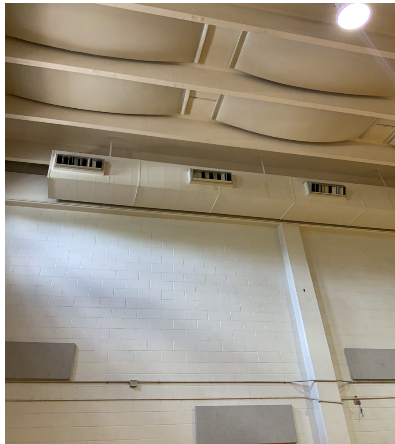
Grille vanes are broken.
