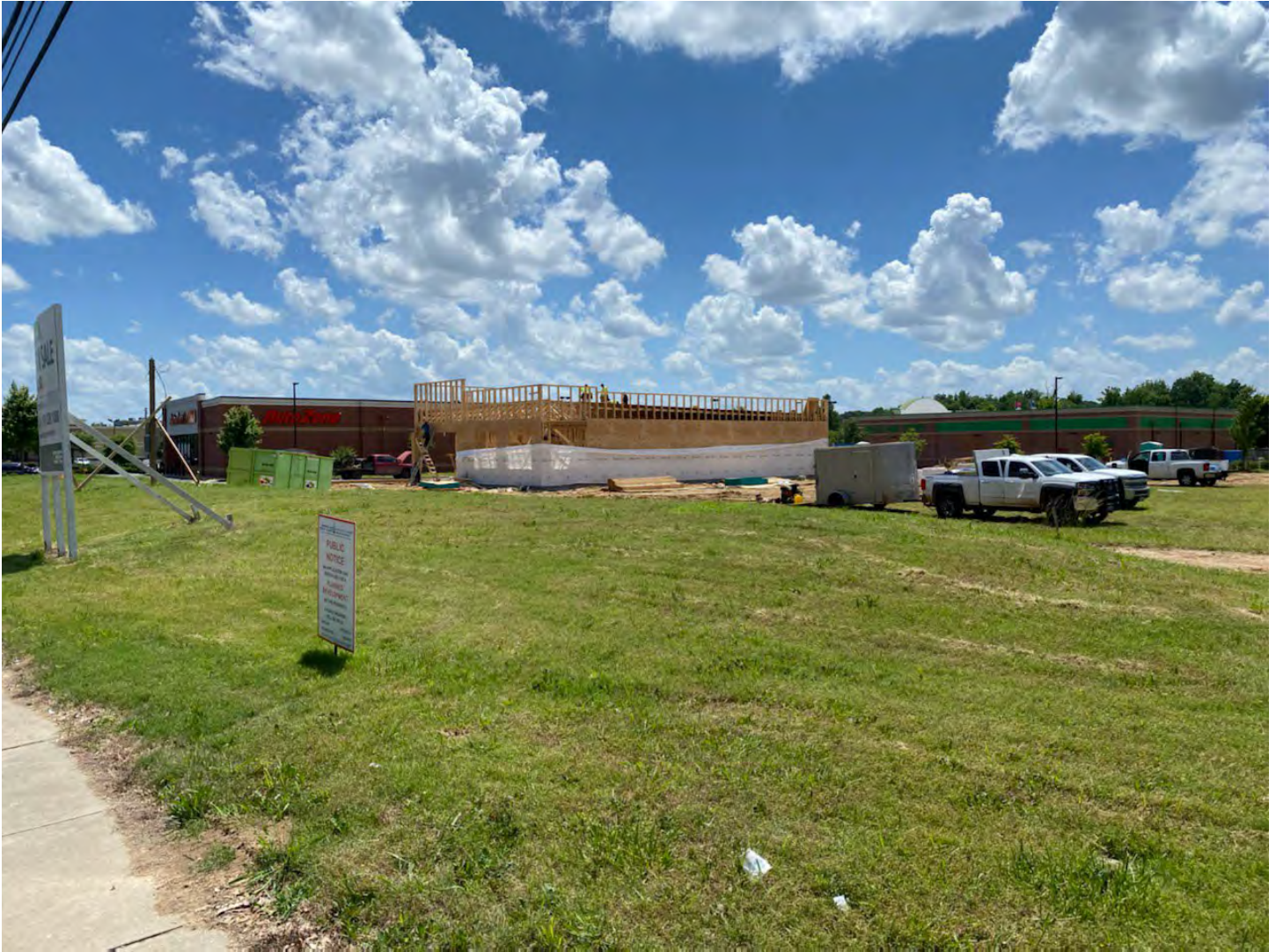
View of adjacent clinic under construction, as well as dollar store and vehicle parts store
