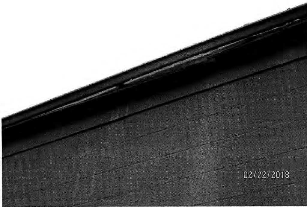
Deferred maintenance – gutters
