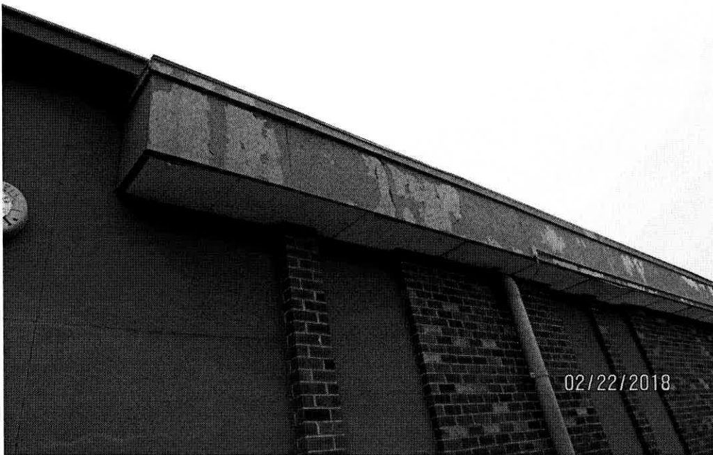
Deferred maintenance – exterior paint
