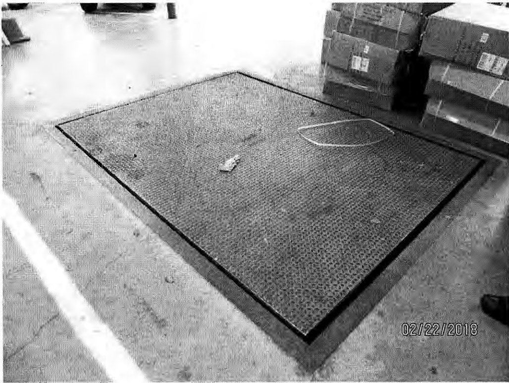
Hydraulic lift in spare motor bay
