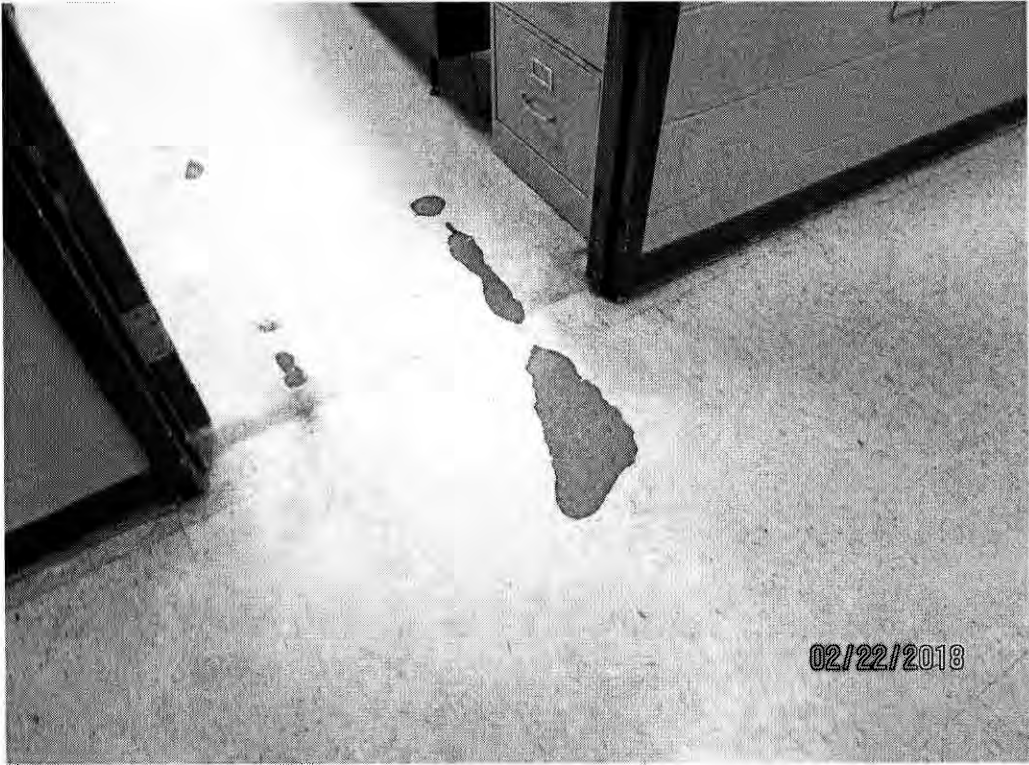
Deferred maintenance – flooring
