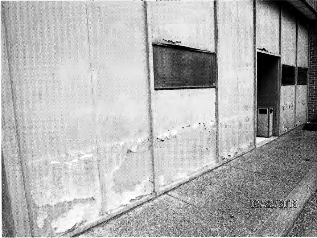
Deferred maintenance – siding
