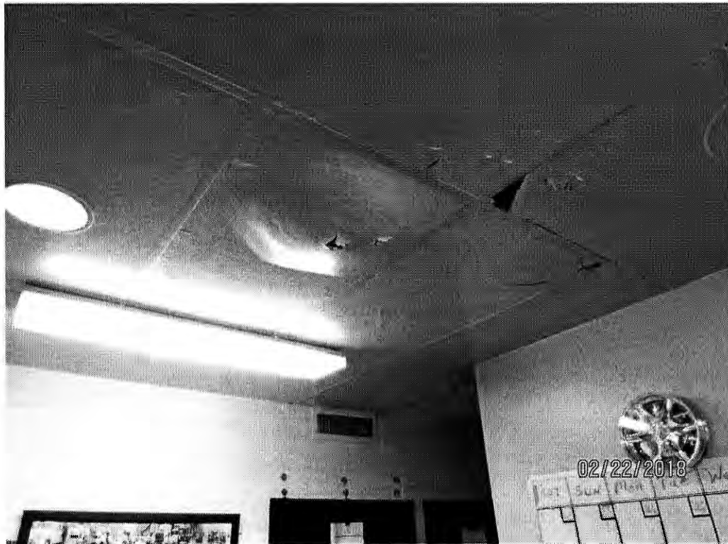
Deferred maintenance – ceiling
