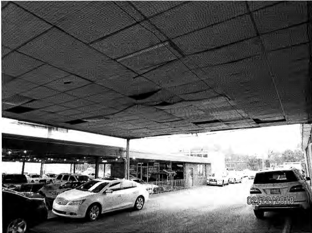
Deferred maintenance – exterior ceilings
