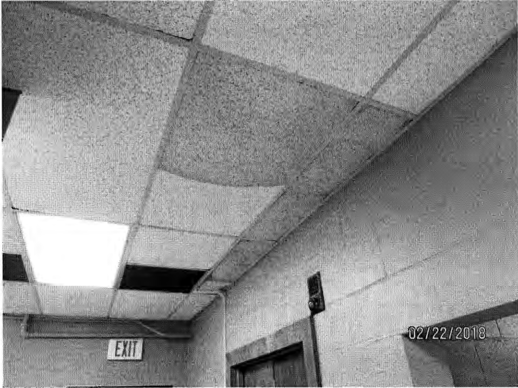
Deferred maintenance – ceilings
