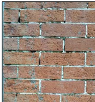
Image 72: This photograph illustrates the negative effects of sandblasting which never should be used to clean brick buildings. Sandblasting will not only erode mortar but will also remove the glazed outer surface of brick, leaving a dimple texture.
