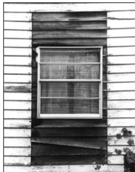
Image 74: The metal window is an obvious replacement for a much larger window that has been removed and the opening has been filled is not appropriate.
