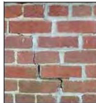
Image 73. The spot repointing of this wall does not match the original in color, texture, or form of joints. The dark gray color and texture of the mortar indicates that Portland cement mortar was used. The cracked and spalled brick (center top) resulted from the expansion of the harder Portland mortar.
