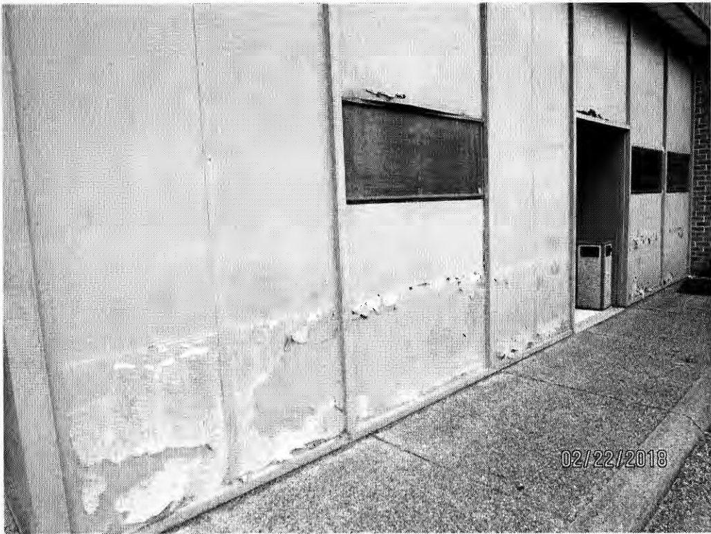
Deferred maintenance – siding
