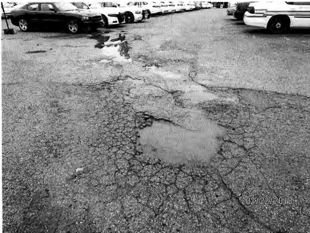
Deferred maintenance – parking lot
