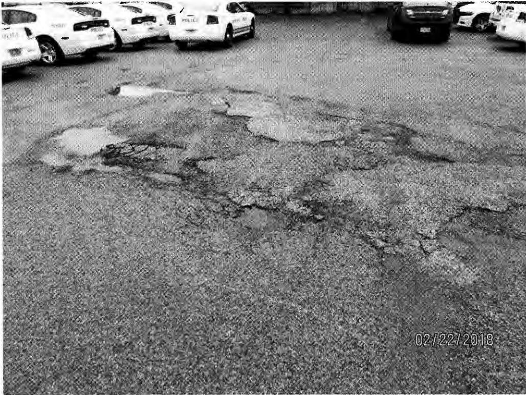
Deferred maintenance – parking lot
