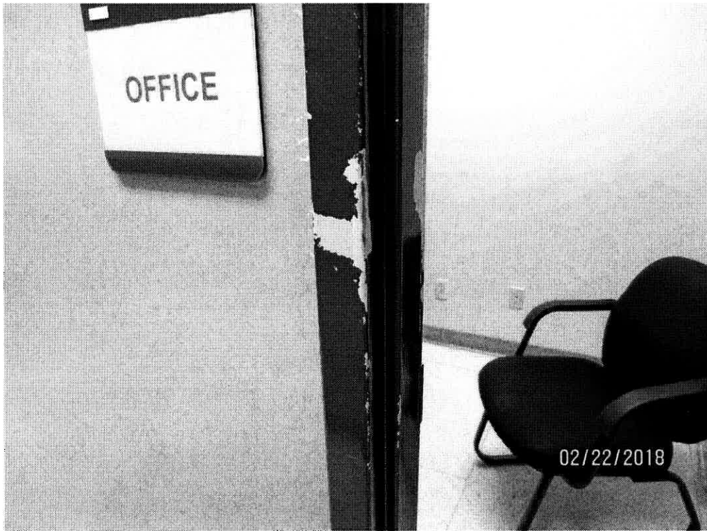
Deferred maintenance – interior paint
