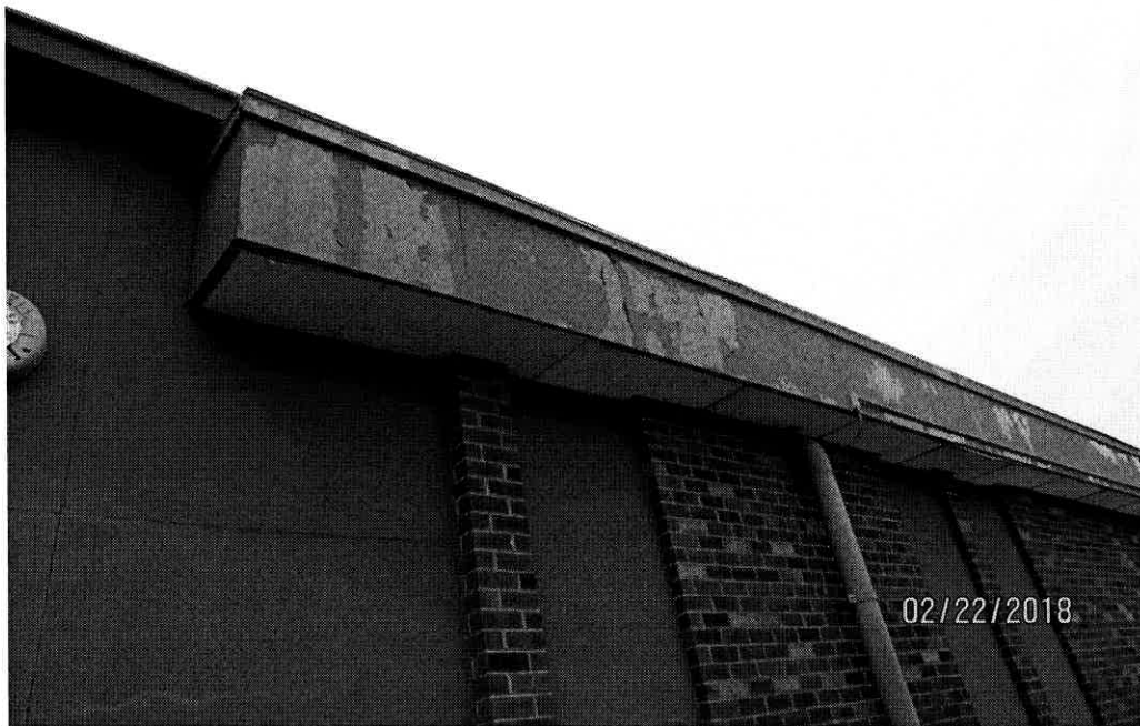
Deferred maintenance – exterior paint
