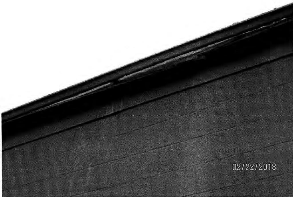
Deferred maintenance – gutters
