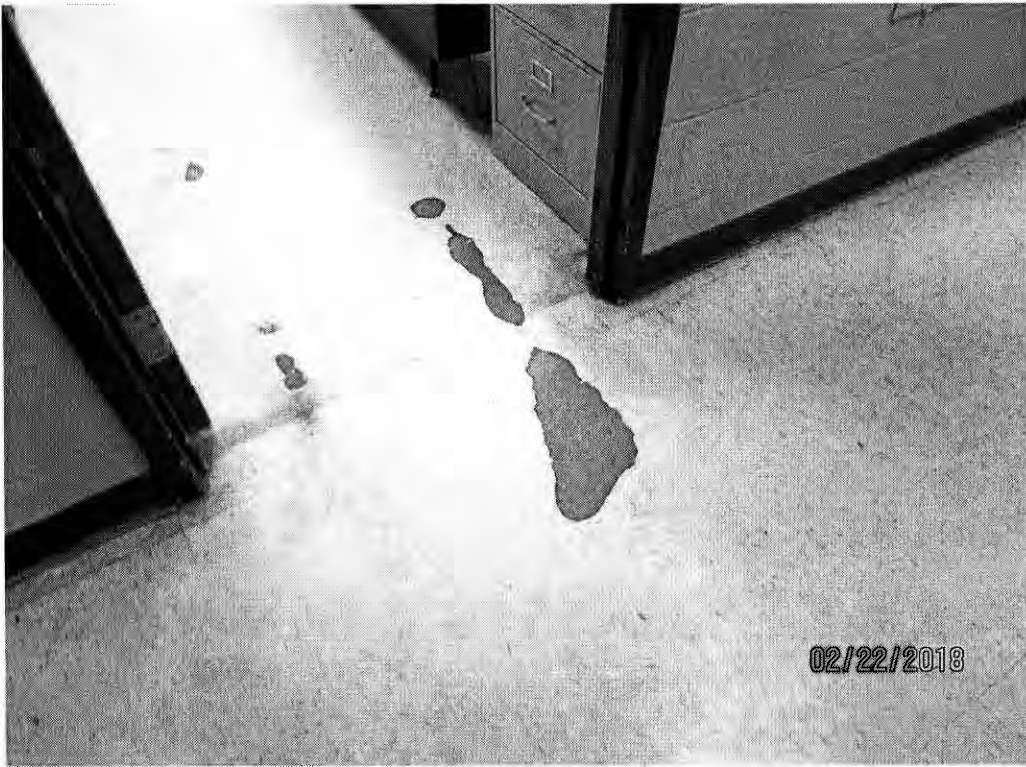
Deferred maintenance – flooring
